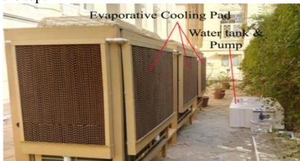
Figure 2 Evaporative Cooling Through Pad
