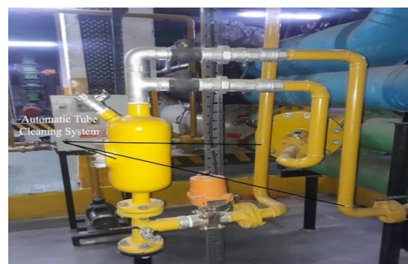
Figure 4 Automatic Tube Cleaning System
